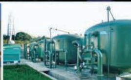
State-of-the-art water treatment plant
